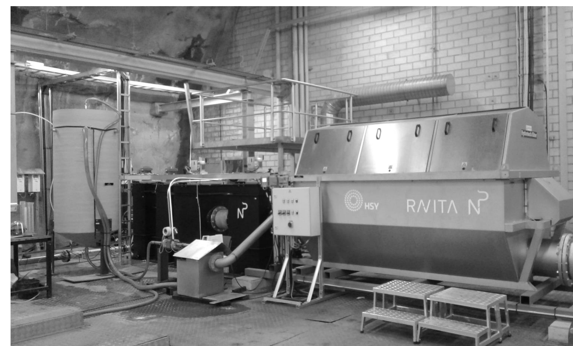
Fig 2. Pilot plant at Viikinmäki wastewater treatment plant in Helsinki
