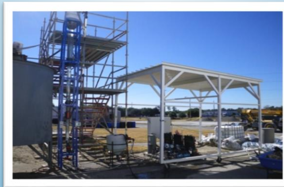
Phosphorus recovery station
