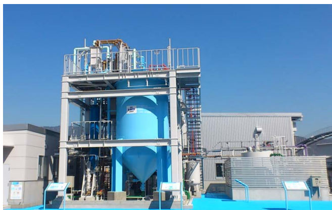
Full-scale plant: struvite recovery demonstration facility of National Institute for Land and Infrastructure Management, which was installed as a part of B-DASH project supported by Ministry of Land, Infrastructure, Transport and Tourism.
