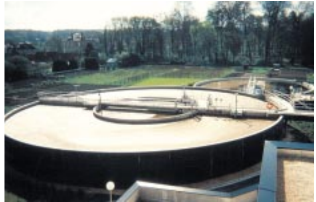
Biological phosphorus removal at Laon sewage works (North East France), Lyonnaise des Eaux. Capacity 40,000 pe.
