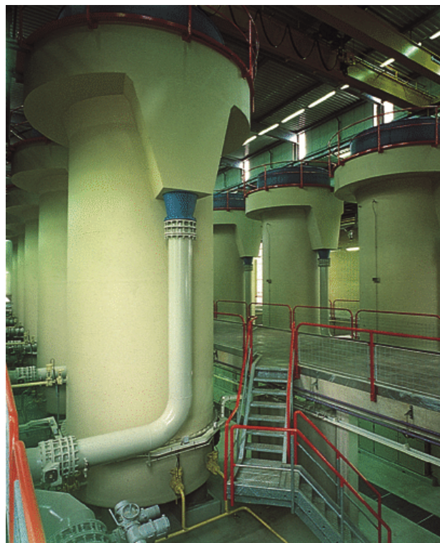
Pellet reactor for nickel and aluminium recovery, Shell Chimie, Berre, France
