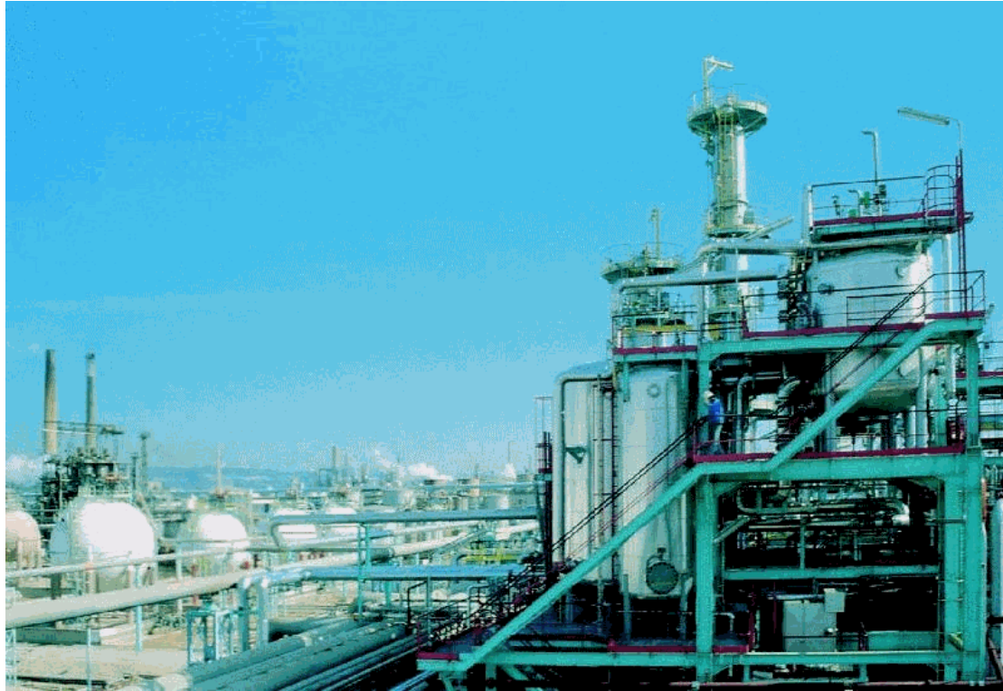
Pellet reactors for softening of drinking water, Municipal Drinking Water Company of Amsterdam, The Netherlands Capacity: 8,500 m 3 /h
