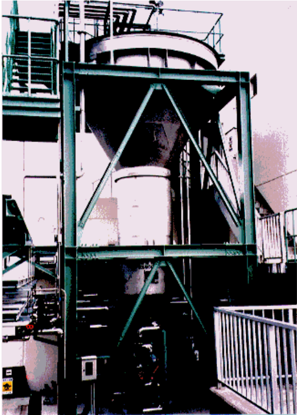
Latest "PHOSNIX" Plant built in 1998 for Sewage
