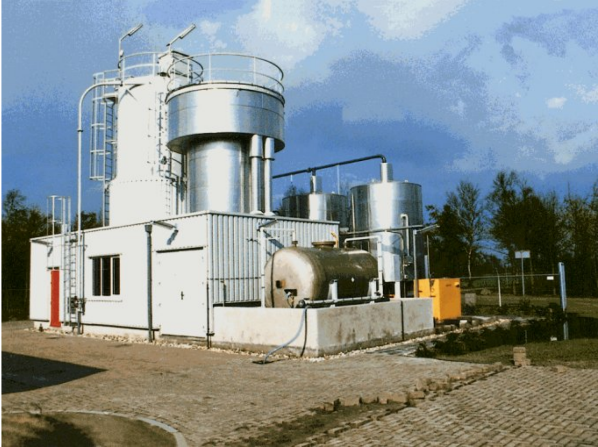
Phosphate removal plant Westerbork
