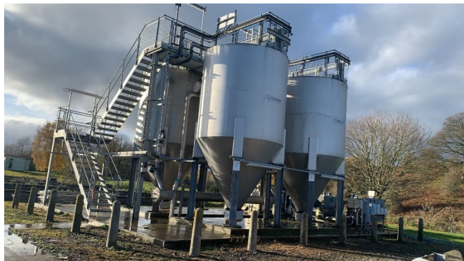
P-removal tertiary filters at Llanberis Welsh Water waste water treatment works (Brightwork, Sand Cycle).
