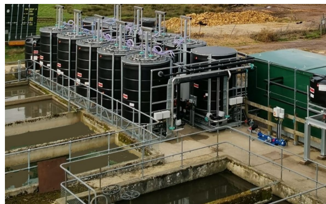
Photo: Broadwindsor Wastewater Treatment Plant, South West Water, UK. - The black tanks are the I-PHYC algae system, the concrete ponds are sludge holding tanks (not related to the algae process).
